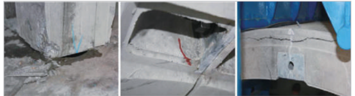
Cracks and damages of rebar reinforced segment
